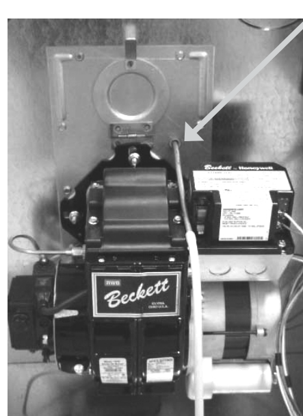
Over-fire draft access port.
