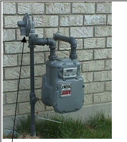
FIGURE 2: GAS REGULATOR VENT
